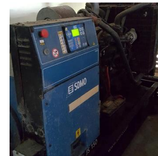
Testing generator at Butler Dairy
